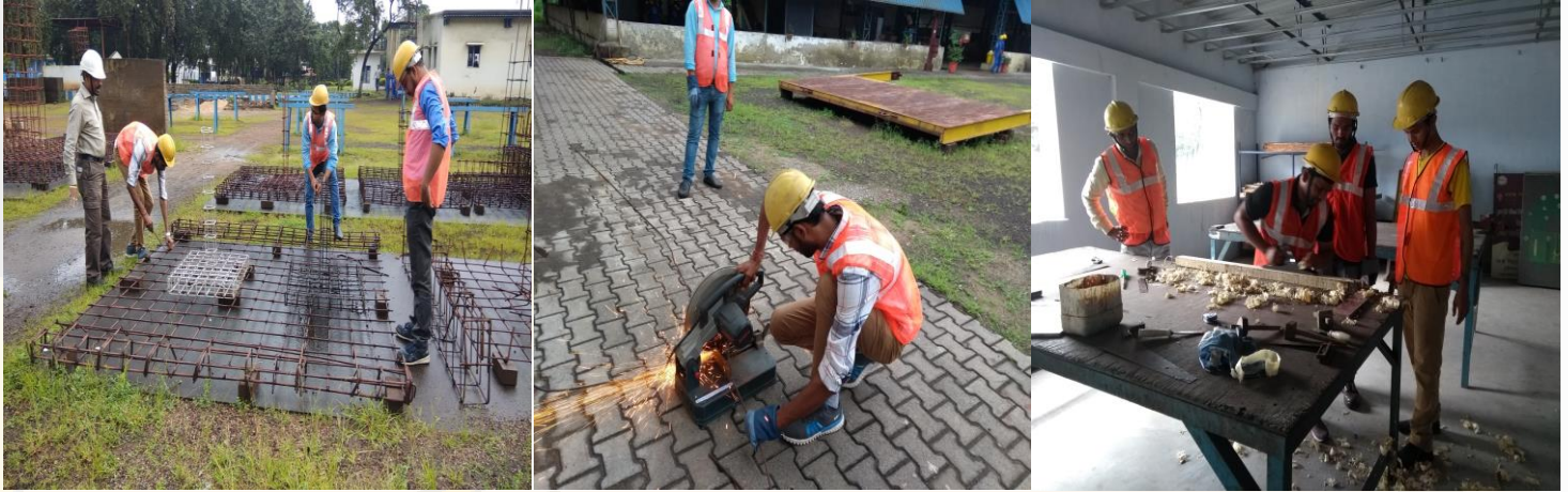
TOT- Bar Bender & Steel Fixer, Shuttering Carpenter-System, Scaffolder-System (Trainer/Assessor) program being conducted at OPJCC Raigarh
