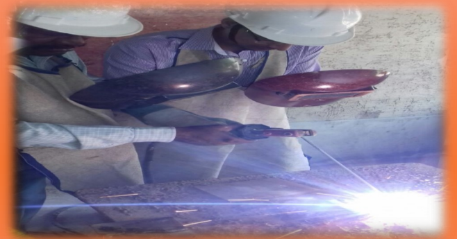
First training program on Fabrication Occupation NSQF L-4 was launched at NAC, Hyderabad
